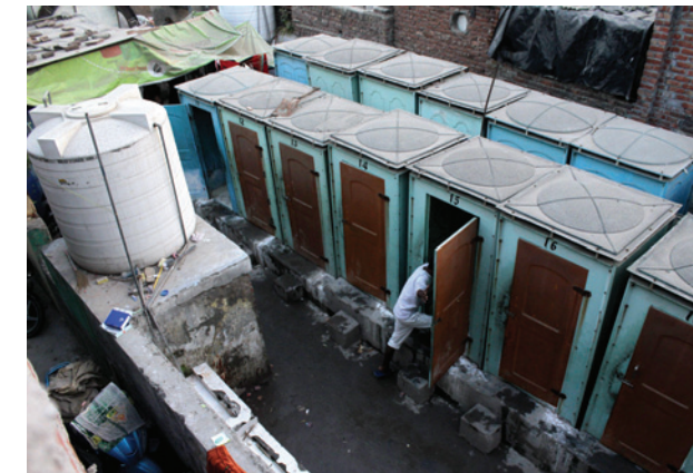
6.4.8 Communal toilet facility in Taimoor Nagar, New Delhi, India. While basic, such facilities greatly enhance the wellbeing of people living in informal settlements.
