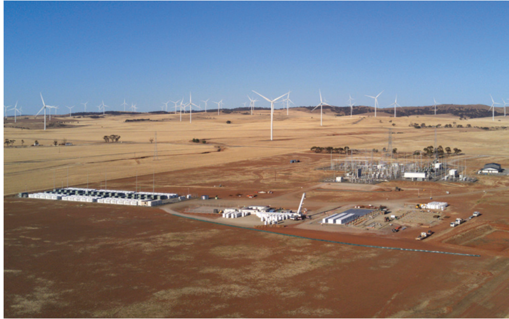
5.4.3 The Tesla 100MW 'big battery' at the Hornsdale Wind Farm, South Australia
