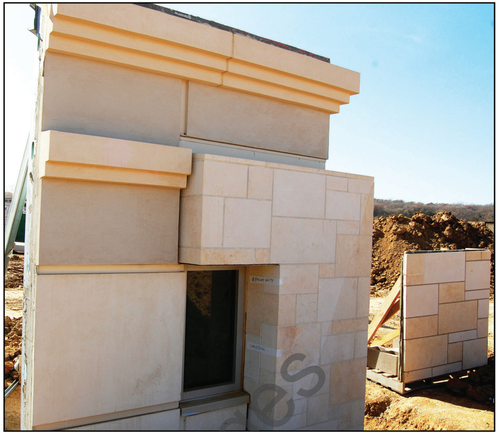
FIGURE 1.16 A typical mockup showing various finishes on the exterior facade of a building under construction. The workmanship in the finished building will be evaluated to match that of the approved mockup.
